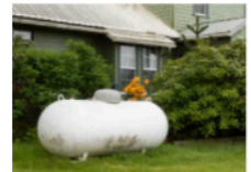
LP Gas Storage
