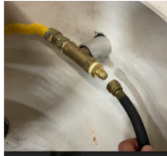
Gas Supply Line to the Ball Valve
